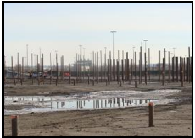
Piling pipes around the site before the surcharge (soil fill) is placed
