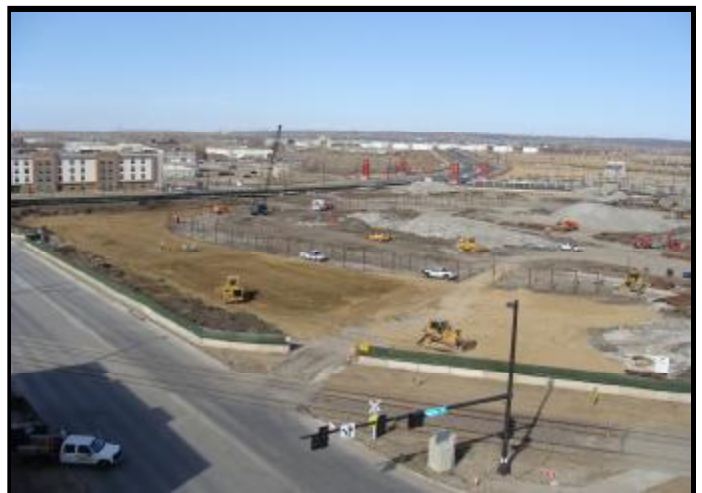
Surcharge Placement in Areas Requiring Soil Fill to Support the Concrete Floors
