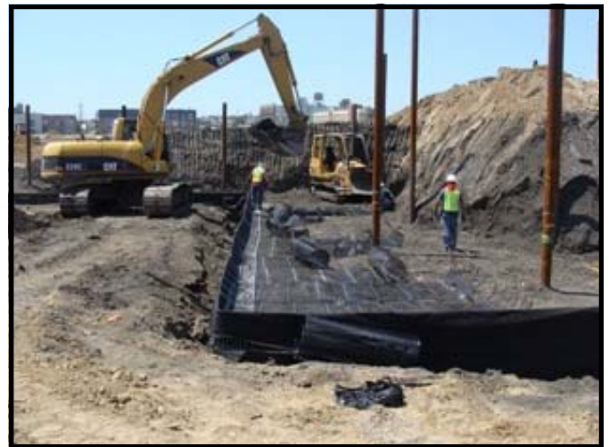
Construction of the bottom portion of the MSE walls in the outfield
